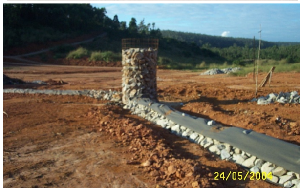
Figure 5. Base Layer Leachate Drains/Venting Wells
