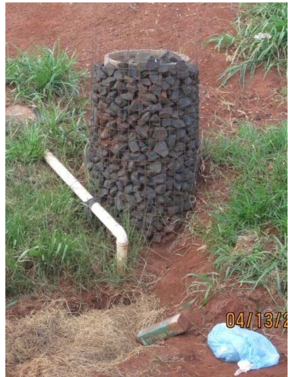
Figure 9. Venting Well with Cage
